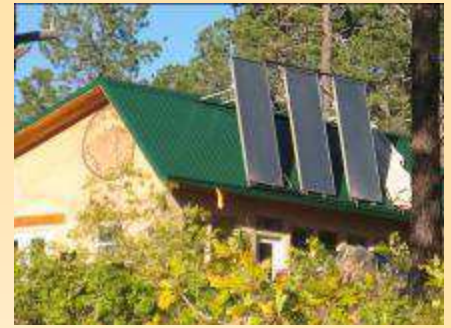
Solar panels on the CI Building
